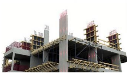
Civil Structure Health and Safety Monitoring
